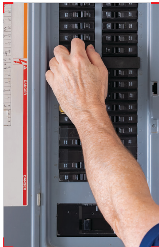
Electrical Circuit Breaker
